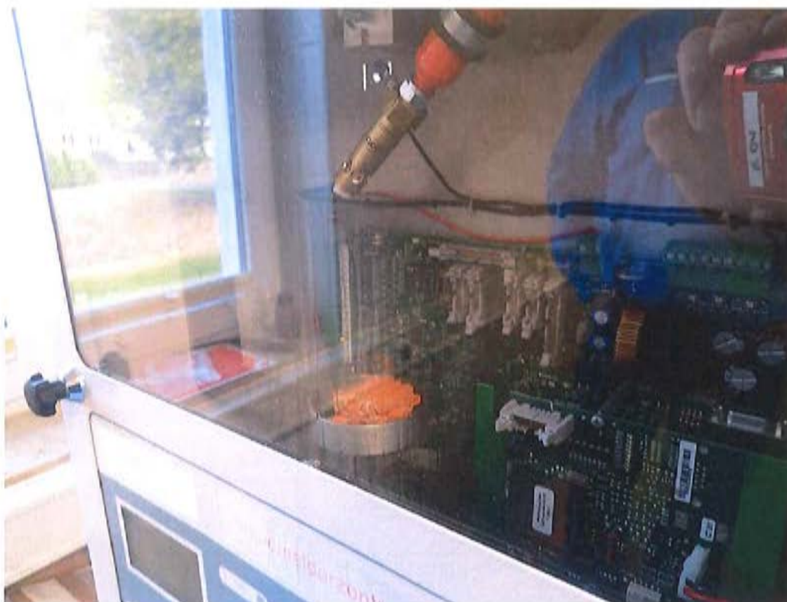
Fig. 21: System has triggered and extinguished, traces of extinguishing medium fluid clearly recognisable on the FACU viewing window
