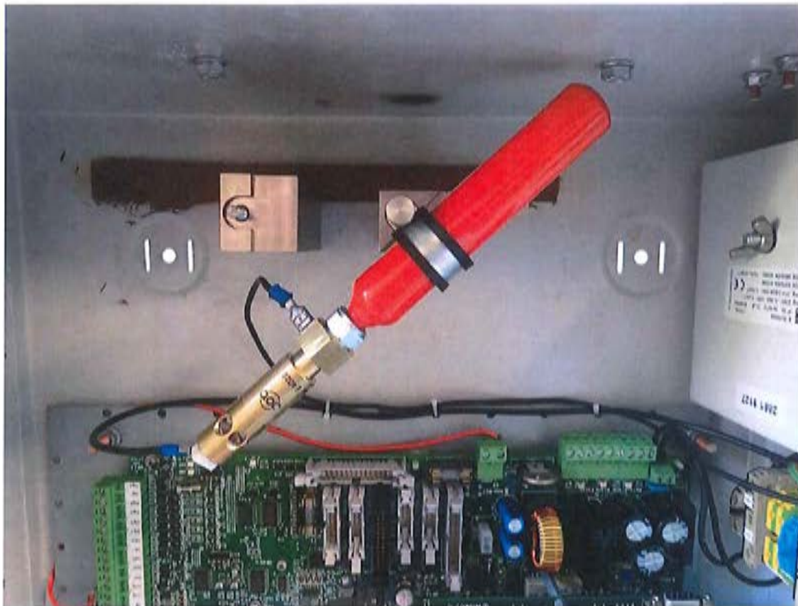
Fig. 17: Arrangement of the AMFE mini extinguisher in the FACU (standard for all tests)
